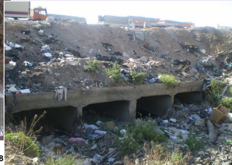
A branch of the river and seemed completely dry, which accumulate dirt, Sep 2007
