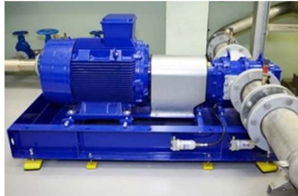
Figure 5 Pressure Reduction Turbine (Source: www.zeropex.com )
